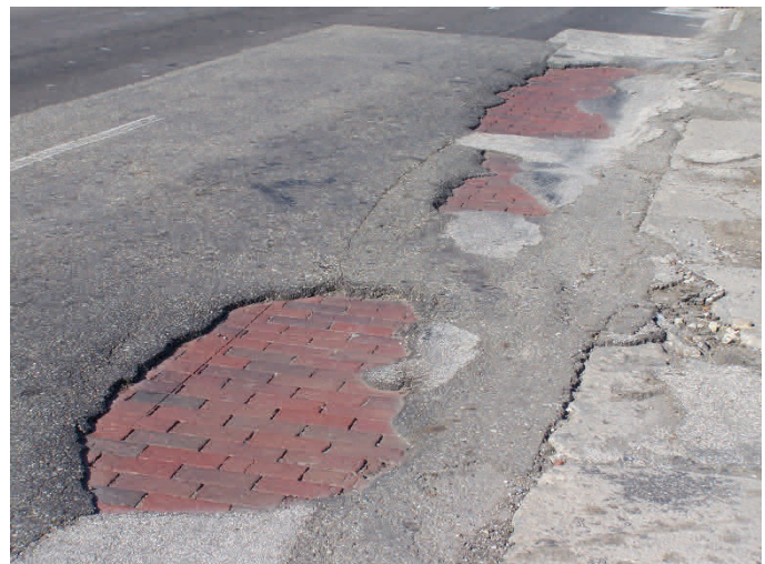
A Street in Need of Resurfacing
