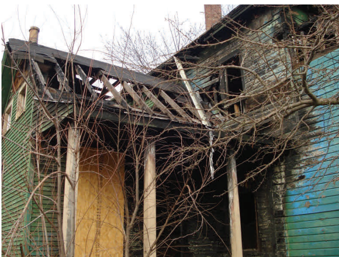
Unsafe Fire Damaged Structure
