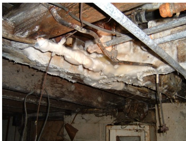
Figure 2. Frozen plumbing and mold growth on floor joists. Note, some of the mold growth is white.
