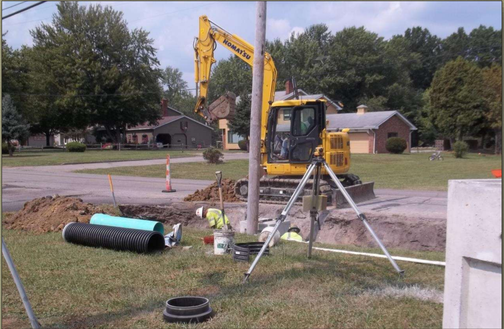
2015 OPWC / CDBG Roads Installing Storm Sewer at Tod Ave & Englesson Dr. NW
