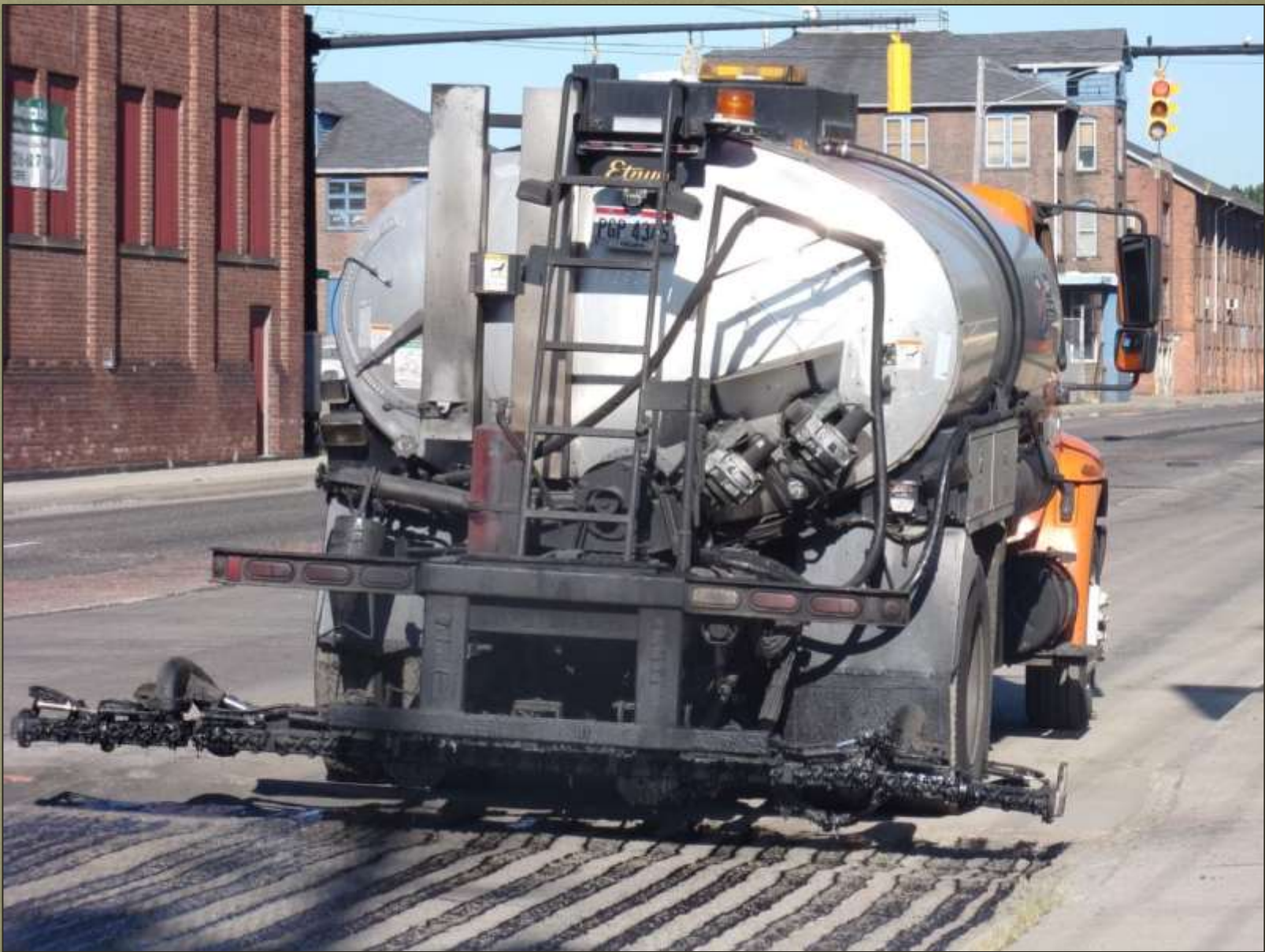
TRU - West Market St - August 3, 2015 East of Austin Ave . - Applying tack before resurfacing with asphalt.
