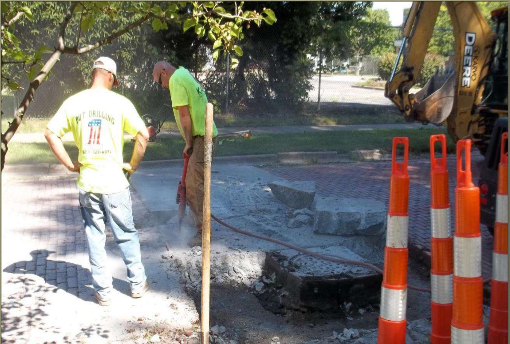
Brick Street Repairs – 2014 City Road Project Jackhammering to remove old concrete – September 2014
