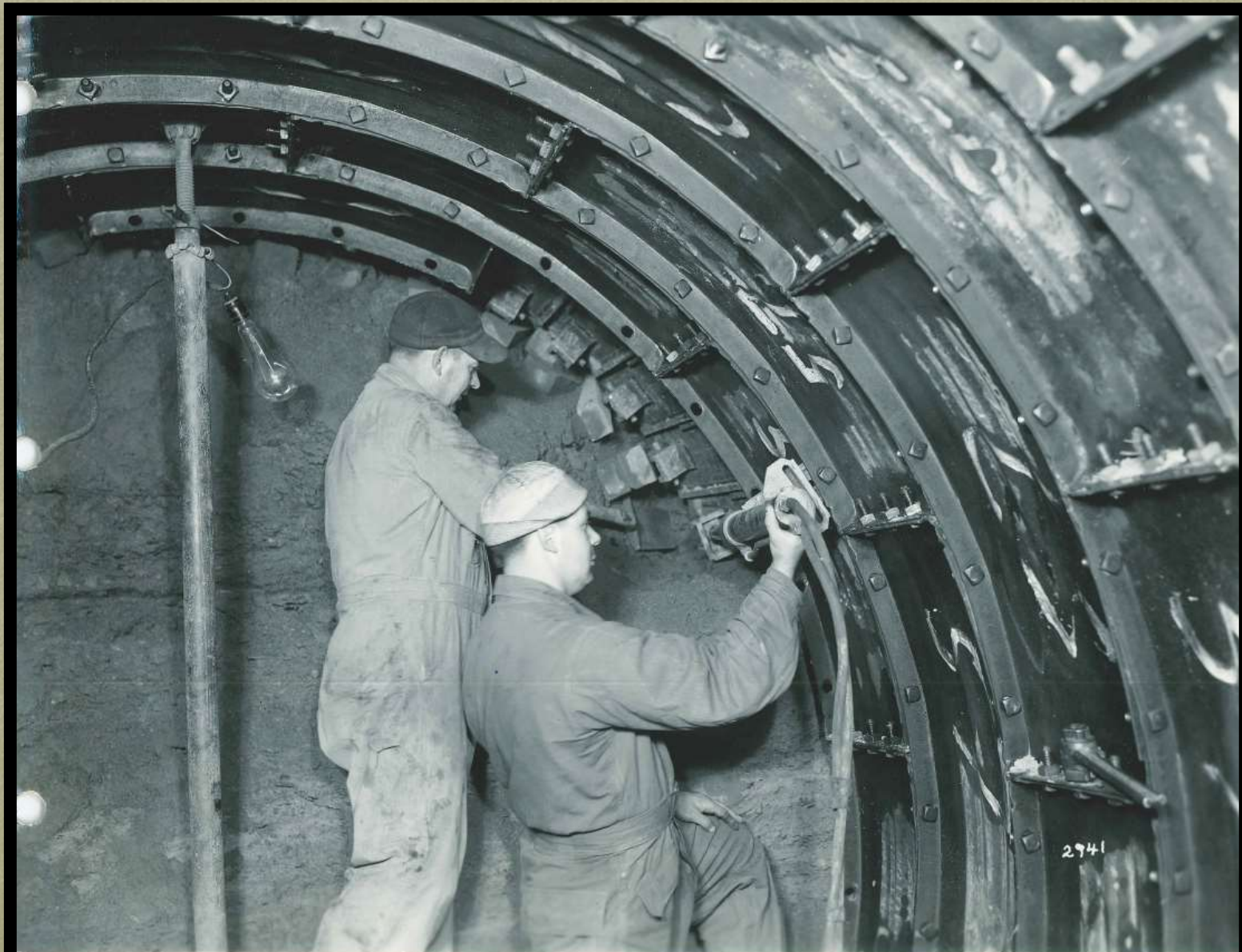
Red Run Combined Sewer (West Branch) - Tunnel Under Erie R.R. (Mainline) - Nov. 194
