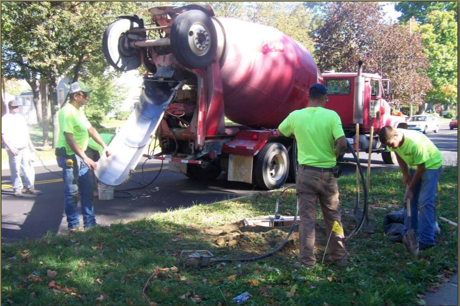
Mahoning Ave Lighting Project – Fall 2010 Pouring concrete foundation for decorative pedestrian lighting.
